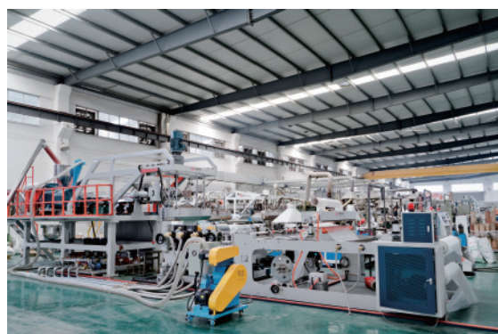
PP流涎机车间 PP Cast film Extrusion Production line
